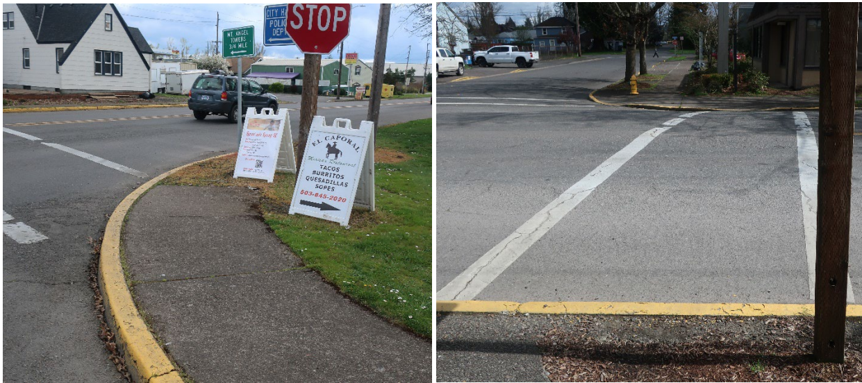
Figure 5. Crosswalks Lacking Curb Ramps Left: Wilco Highway and Church Street. Right: Main Street and Palmer Street.
